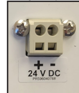
Electrical connection for 24 VDC
